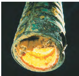
▲ FIGURE 18.22 Scale formation. The interior of this water pipe has been coated with \text{CaCO}_3 and other insoluble salts deposited from hard water.
